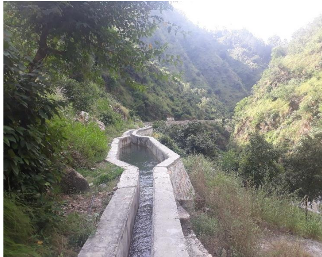
Figure 44: Water channel at MHP plant site, Sar Kalay, Buner district
