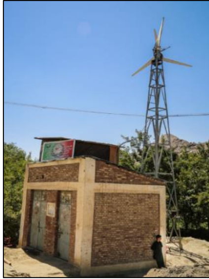
Figure 26: 5 kW Wind Turbine in Sang-E-Nawishta Village of Kabul 20
