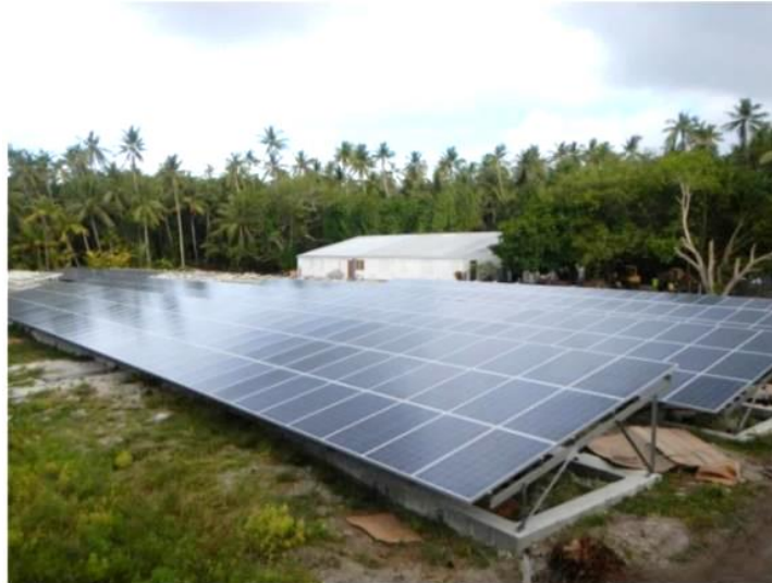
Figure 42: Installed solar PV system in Tokelau 59
