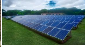
8 Solar Mini grid Projects in Operation
