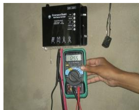
Charge Controller Checking
