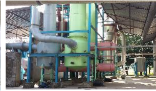
Financed 1 Biomass Based Power Projects
