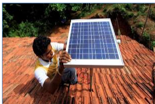
Solar Panel Checking
