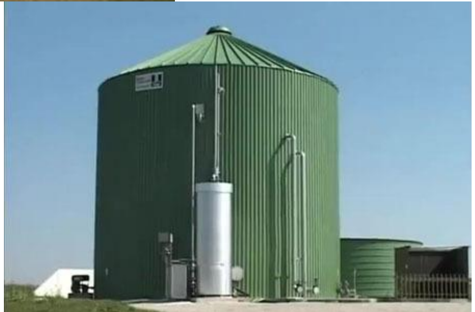
UASB Reactor. Porur, Chennai, India
