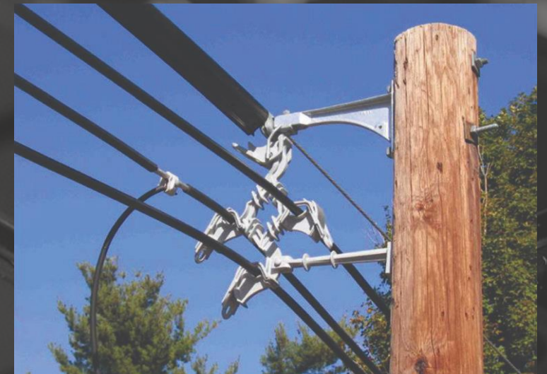
3. Covered Conductor (CC)
