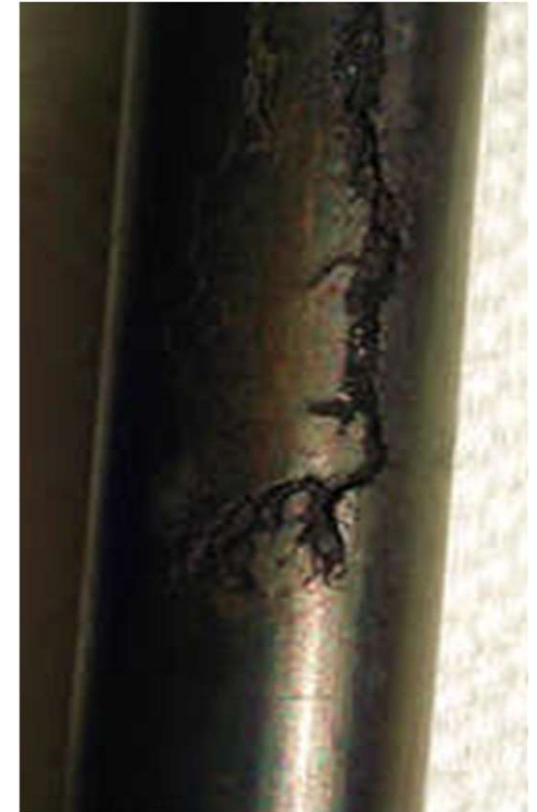
Surface tracking & polymer Erosion due to High Voltage
