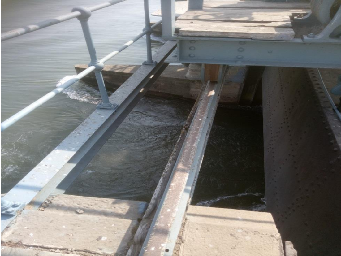
Annexure –III Fig: 0-3: Exact location for the installation, 2nd option at the entrance of 2nd channel under the bridge.
