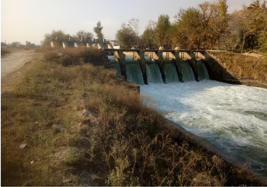
Figure 0-3: View of the Machai canal showing the steps created to decrease the velocity of water
