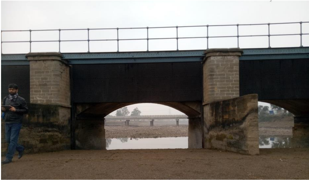
Annexure –III Fig: 0-7: Channel No.7 under Jaggu head works bridge, after annual shut down, which is a final selection for installation of turbine.
