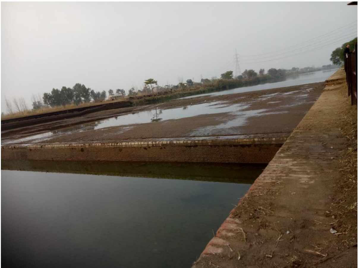
Annexure –III Fig: 0-6: A siphon near Jaggu Head Works, a proposed location for the installation of turbines.
