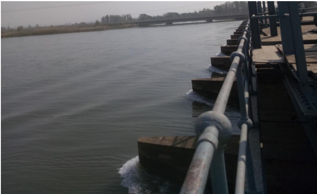
Annexure –III Fig: 0-4: Front view of the bridge showing 17 channels of the canal.
