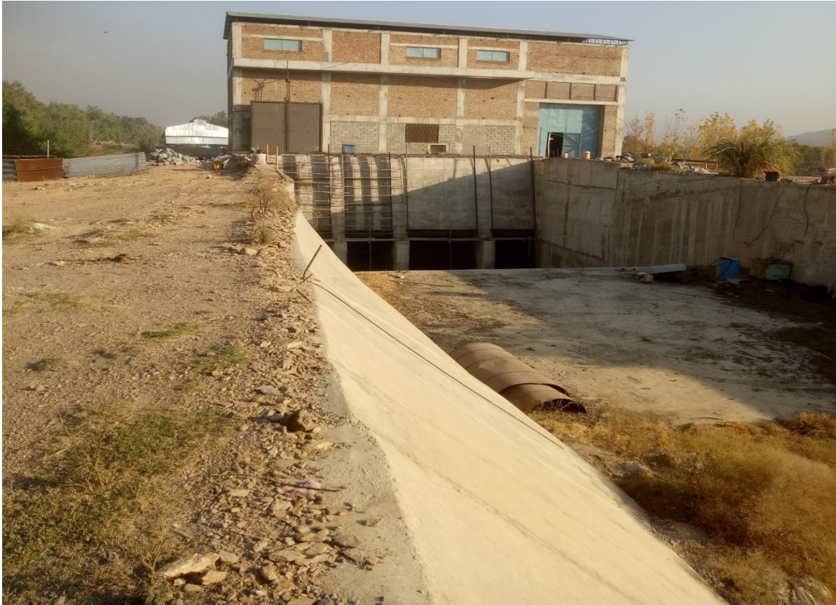
Annexure- II Fig: 1-6: Another 2 MW hydropower project under construction on Machai canal
