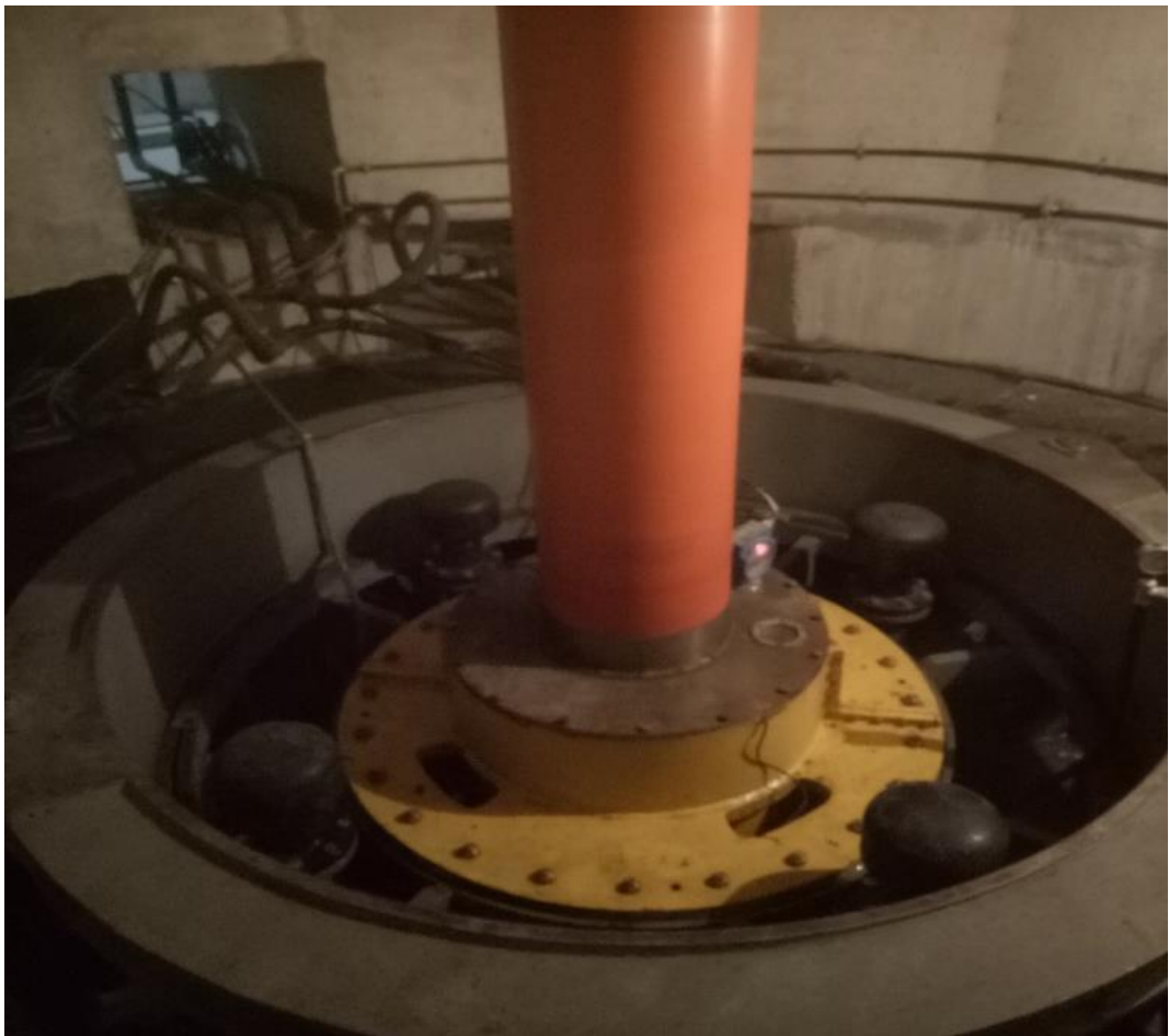
Annexure- II Fig: 1-4: Turbine room of the 2.6 MW Machai Hydropower Project
