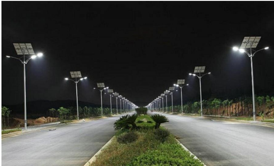
Figure- 12: Solar Street Lighting of Chirirbandar roads, Bangladesh 14
